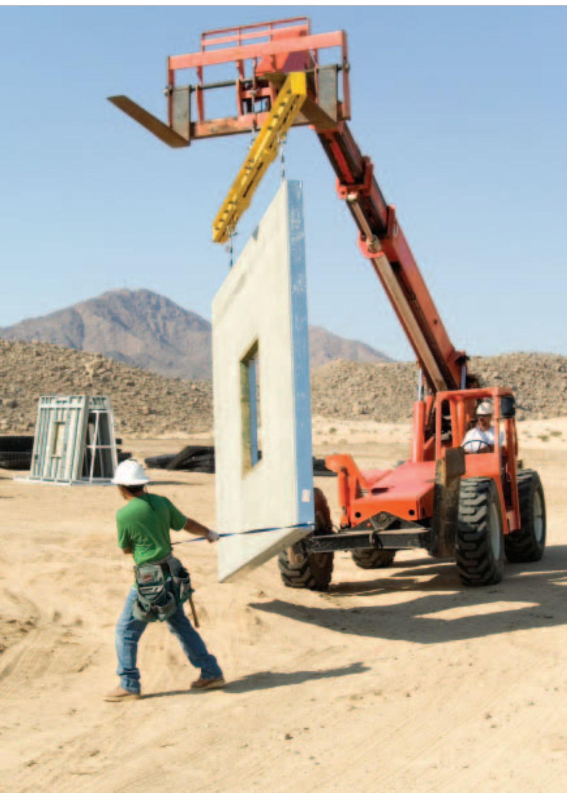
◀ A lightweight forklift is all that is required to place the wall panels.
